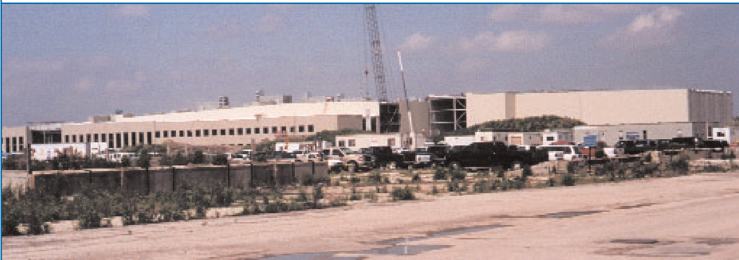
Photo of Triumph Foods new St. Joseph, Missouri pork processing facility under construction. This is the largest pork processing plant (680,000 square feet) to be built in the U.S. in over eight years, and utilizes all Jarvis Products equipment. Besides processing operations, the site will house Triumph's corporate headquarters.
